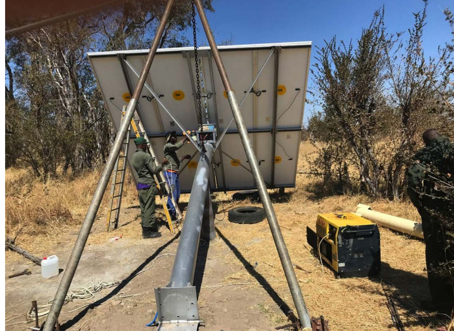
Solar Array going up at Kennedy 1
